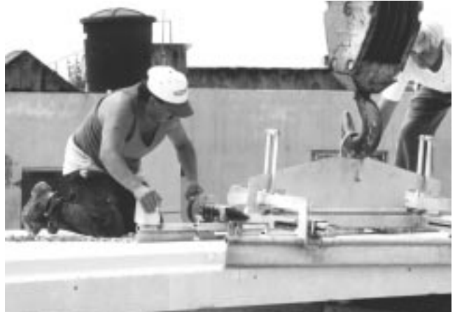
Fig. 10: Place the panel according to guidelines on top of support elements, open the buckets and remove the lifting gear.
