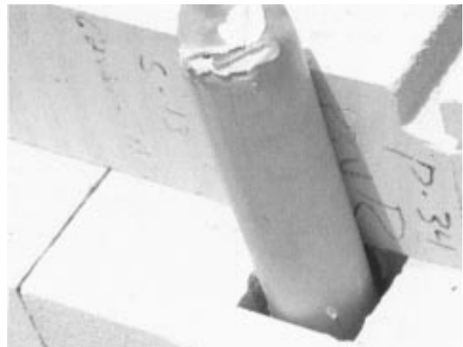
Fig. 17: Pipe lines through sContec walls.
