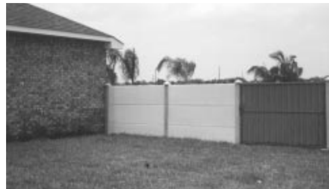
Fig. 10: Gate in Contec Fence System.
