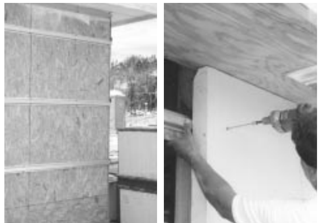
Fig. 8: Once furring channels and asphalt felt are placed, fix Contec Board using proper screws (see screws specifications tables).
